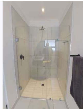
Ref # 19.4 - Shower door is too small and needs to be replaced
