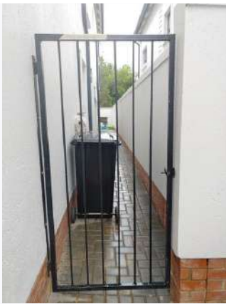
Ref # 23.4 - Gate rusted in places
