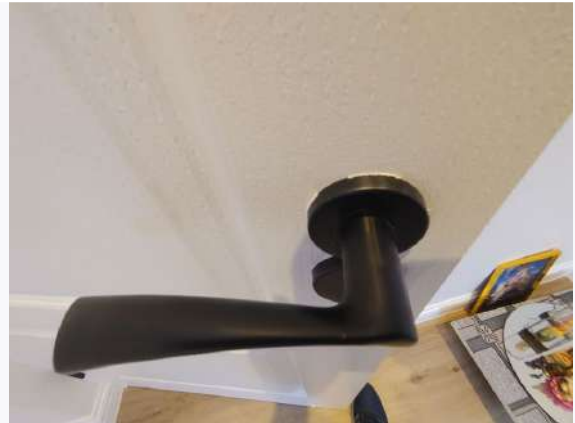
Ref # 13.2 - Paint splatter and scuff marks on the door lock sets
