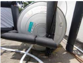
Ref #6 - Electric Geyser with Tank
