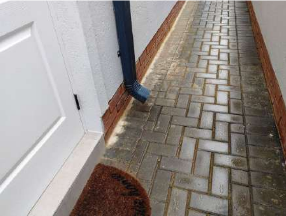
Ref # 23.1 - Downpipes and roof slab drainage is discharging onto unprotected paving at
