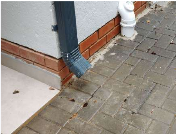
Ref # 23.1 - Downpipes and roof slab drainage is discharging onto unprotected paving at
