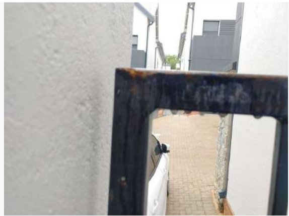
Ref # 23.4 - Gate rusted in places
