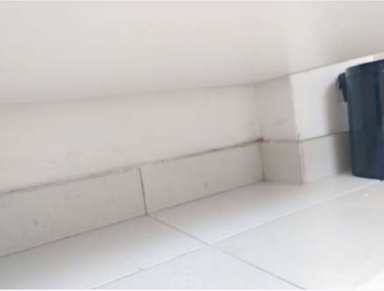
Ref # 18.1 - Untidy finishing
