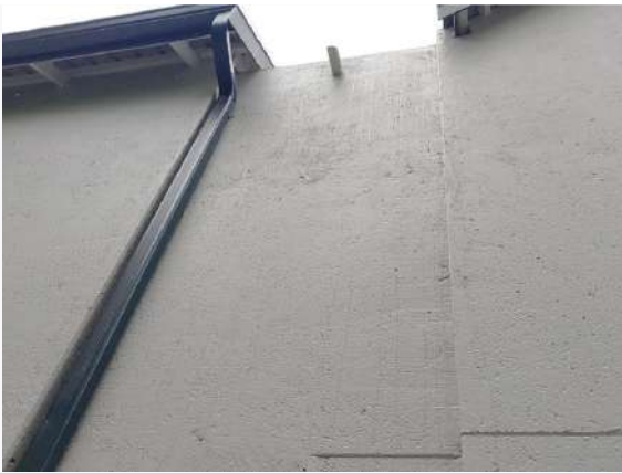
Ref # 23.1 - Roof slab drainage is discharging onto unprotected paving at the base of th
