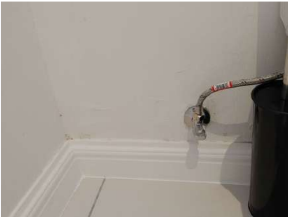
Ref # 21.1 - Active rising / lateral damp measured
