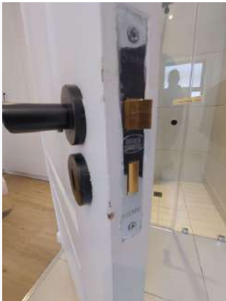
Ref # 11.3 - Paint splatter and scuff marks on the door lock sets
