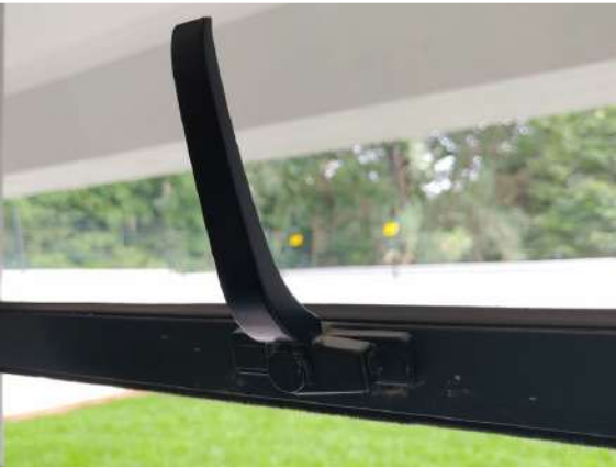
Ref # 15.2 - Window opener loose and requires adjustment
