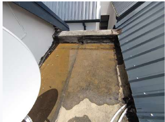
Ref # 4.1 - Water ponding on slab
