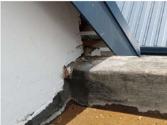
Ref # 4.2 - Areas not waterproofed
