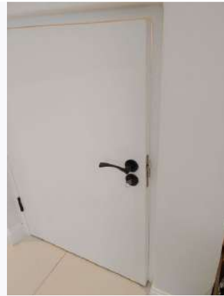
Ref # 15.3 - Door not closing properly
