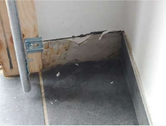
Ref # 22.4 - Tiled skirting missing
