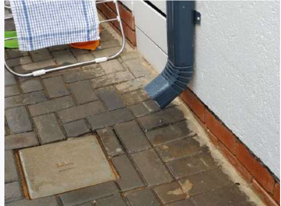
Ref # 23.1 - Downpipes and roof slab drainage is discharging onto unprotected paving at
