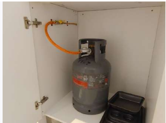
Ref # 8.2 - No provision made for ventilation
