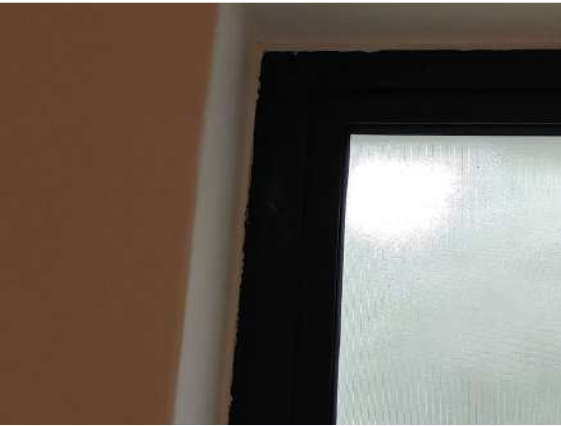
Ref # 21.2 - Untidy painting and finishing
