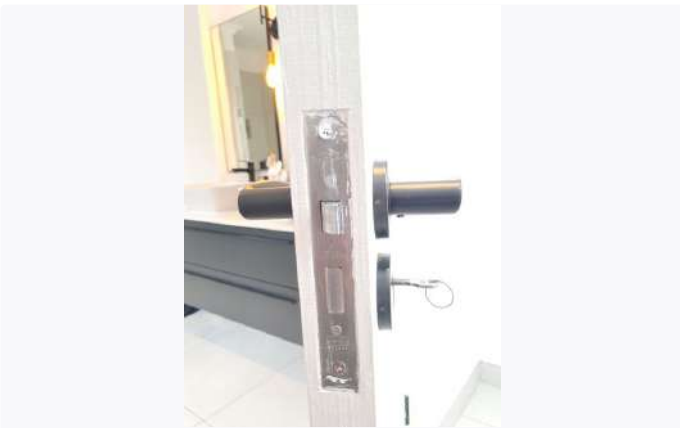
Ref # 18.3 - Paint splatter and scuff marks on the door lock sets
