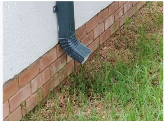
Ref # 23.1 - Downpipes is discharging onto unprotected soil at the base of the wall
