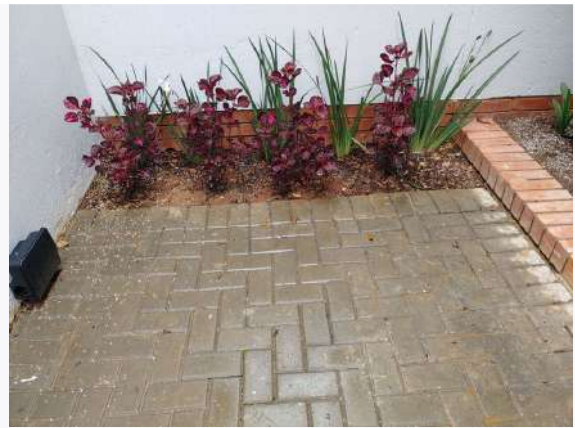
Ref # 23.1 - Evidence of storm water ponding near structures
