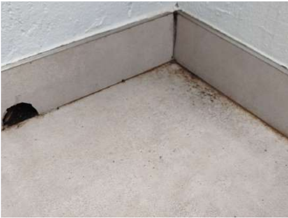
Ref # 10.2 - Areas where water is ponding
