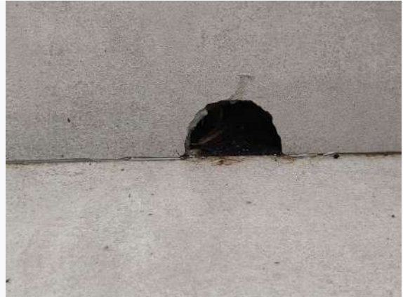
Ref # 10.2 - Drainage outlet appear to be to undersized
