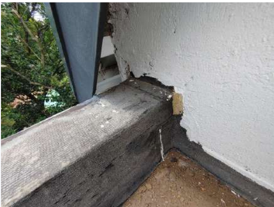
Ref # 4.2 - Areas not waterproofed
