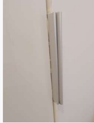
Ref # 16.1 - Untidy finishing
