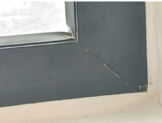
Ref # 18.2 - Gap at mitre joint
