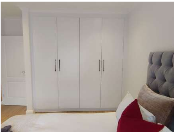
Ref # 12.3 - Cupboard doors and hinges require alignment and/or adjustment
