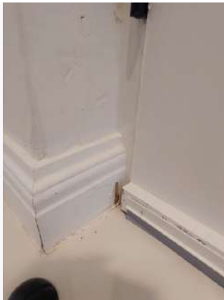
Ref # 15.4 - Door catching on skirting
