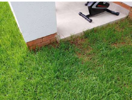
Ref # 23.1 - Roof slab drainage is discharging onto unprotected soil at the base of the
