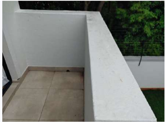
Ref # 10.2 - Top of the masonry balustrades do not appear to be waterproofed
