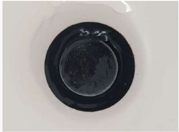
Ref # 20.4 - Pop-up drain plug has scuff marks
