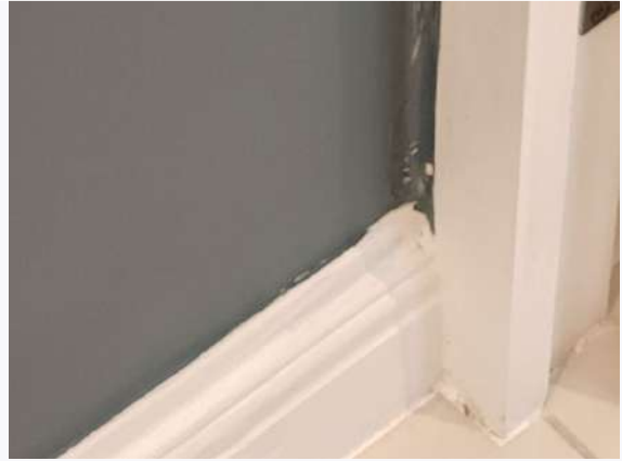
Ref # 15.1 - Untidy painting and finishing
