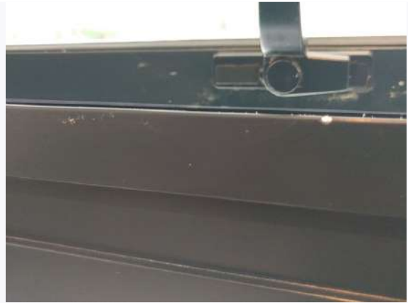
Ref # 15.2 - Window opener loose and requires adjustment
