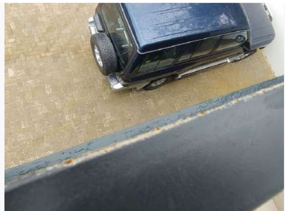
Ref # 12.1 - Rust observed on balustrade
