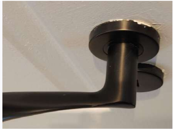
Ref # 21.3 - Paint splatter and scuff marks on the door lock sets
