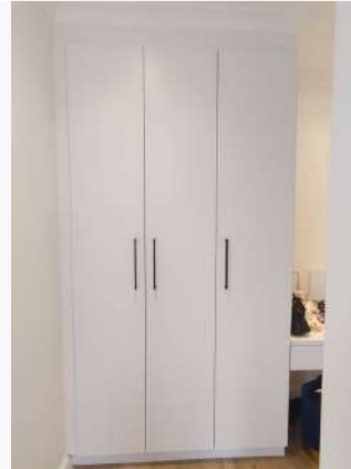
Ref # 10.4 - Cupboard doors and hinges require alignment and/or adjustment
