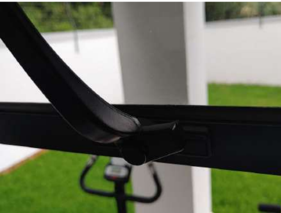
Ref # 15.2 - Window opener loose and requires adjustment
