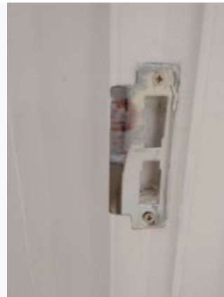
Ref # 10.3 - Untidy installation of striker plate
