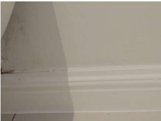
Ref # 21.1 - Active rising / lateral damp measured
