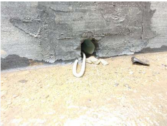
Ref # 4.1 - Drainage outlet is not effective
