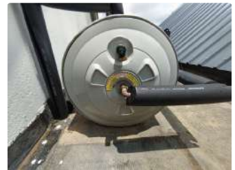
Ref #6 - Electric Geyser with Tank
