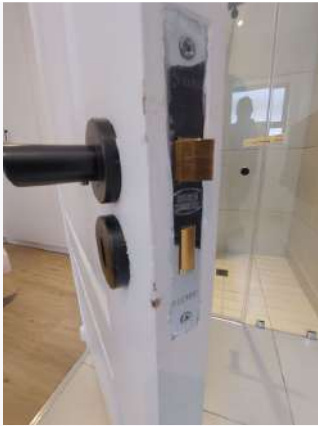
Ref # 19.1 - Paint splatter and scuff marks on the door lock sets
