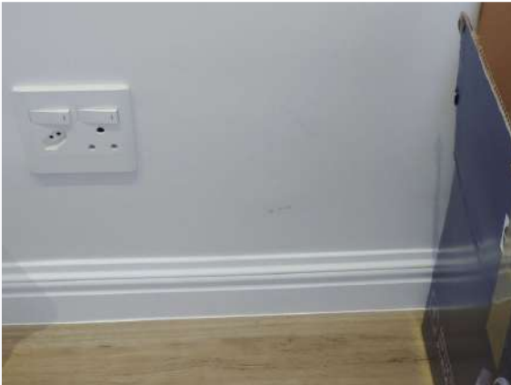
Ref # 13.1 - Scuff marks observed in areas
