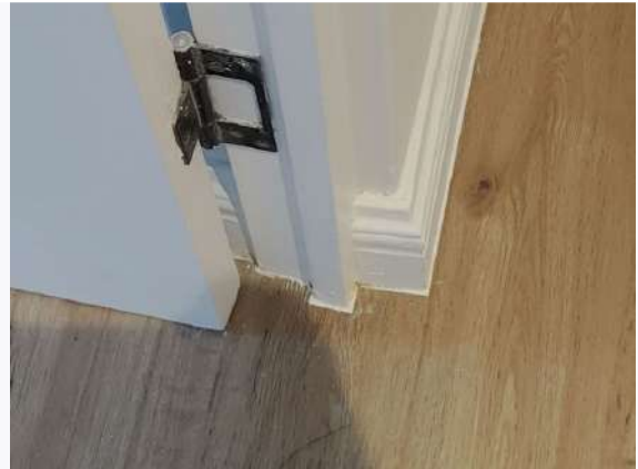
Ref # 14.1 - Untidy finishing at intersection to wall and floor
