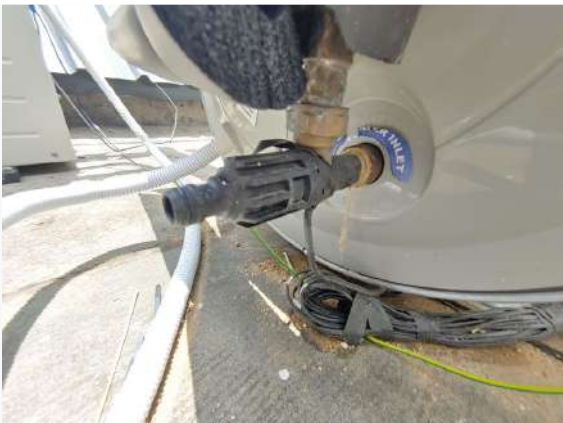
Ref # 6.3 - Electrical insulation tape wrapped around a fitting
