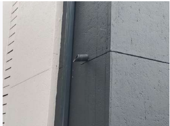
Ref # 23.1 - Downpipes and roof slab drainage is discharging soil at the base of the wal
