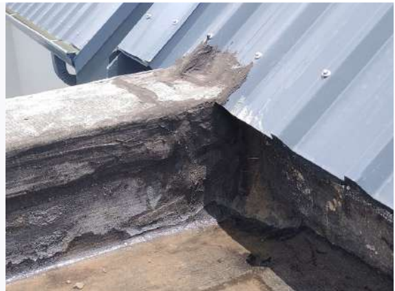
Ref # 4.2 - Waterproofing on parapet wall overlapping onto adjacent metal roof
