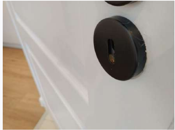
Ref # 19.1 - Paint splatter and scuff marks on the door lock sets
