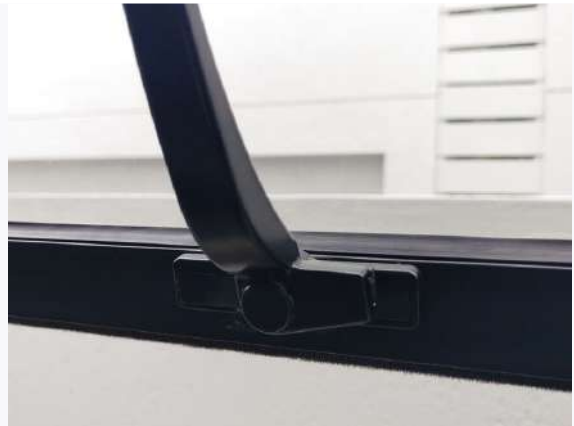
Ref # 15.2 - Window opener loose and requires adjustment
