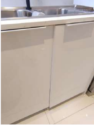
Ref # 16.1 - Door requires alignment
