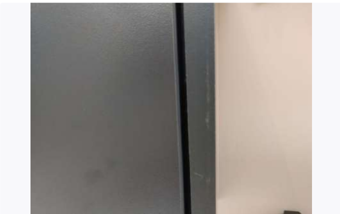
Ref # 18.4 - Paint splatter and scuff marks on the cupboard
