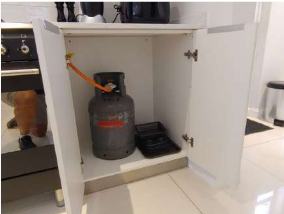
Ref # 16.1 - Floor unit housing the gas bottle is not ventilated
