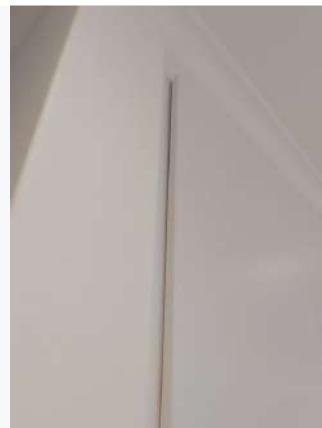
Ref # 12.3 - Cupboard doors and hinges require alignment and/or adjustment
