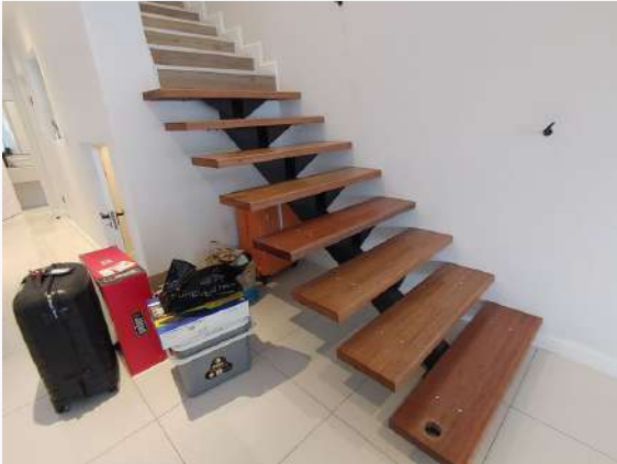
Ref # 17.2 - No balustrades
