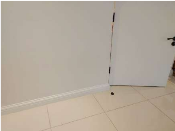
Ref # 15.1 - Active rising / lateral damp measured
