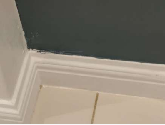
Ref # 15.1 - Untidy painting and finishing
