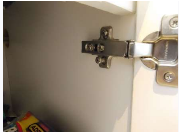
Ref # 16.1 - Hinge is not screwed in properly
