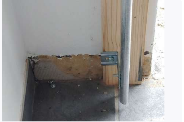
Ref # 22.4 - Tiled skirting missing
