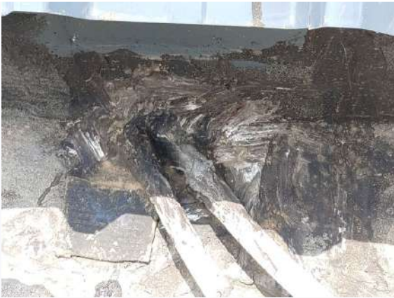
Ref # 4.2 - Projections through the roof slab are not waterproofed effectively
