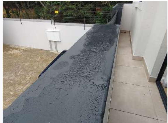
Ref # 12.1 - Top of the masonry balustrades do not appear to be waterproofed
