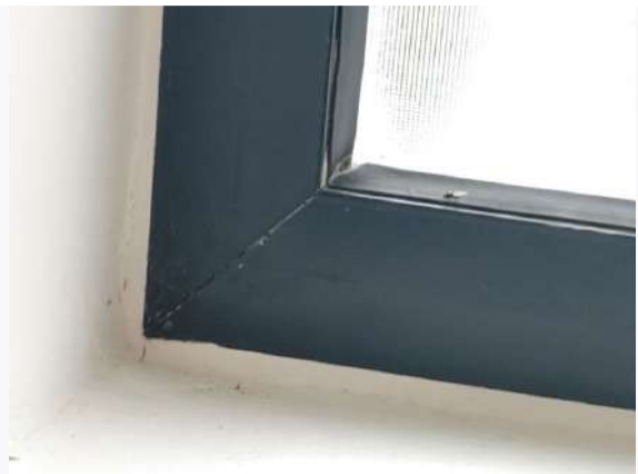
Ref # 18.2 - Gap at mitre joint
