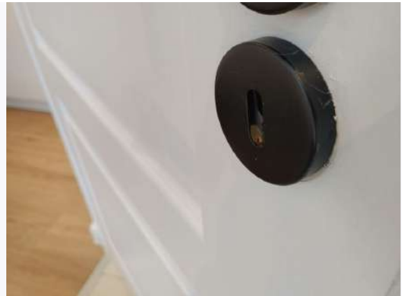
Ref # 11.3 - Paint splatter and scuff marks on the door lock sets
