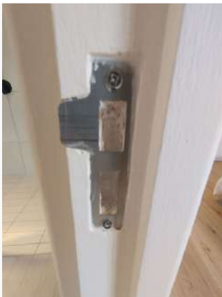
Ref # 20.2 - Untidy installation of striker plate
