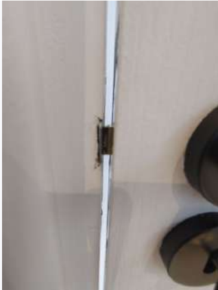
Ref # 20.2 - Door does not close properly
