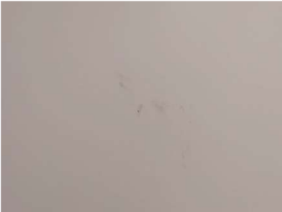
Ref # 11.1 - Scuff marks observed in areas
