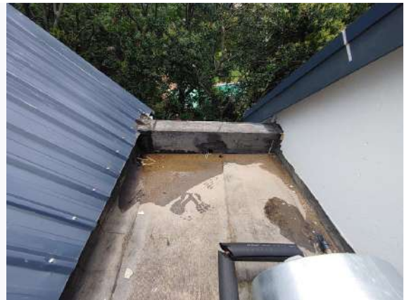
Ref # 4.1 - Water ponding on slab
