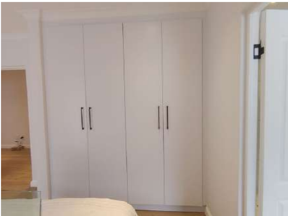
Ref # 11.4 - Cupboard doors and hinges require alignment and/or adjustment
