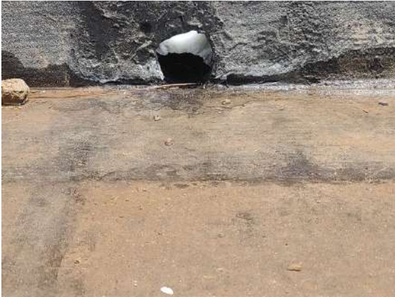
Ref # 4.1 - Drainage outlet is not effective
