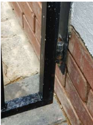
Ref # 23.4 - Gate rusted in places
