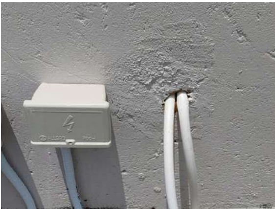
Ref # 2.1 - Untidy finish near geyser
