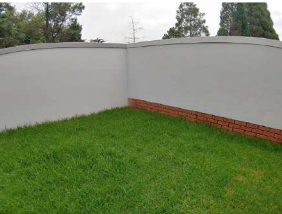
Ref # 23.1 - Evidence of storm water ponding near structures
