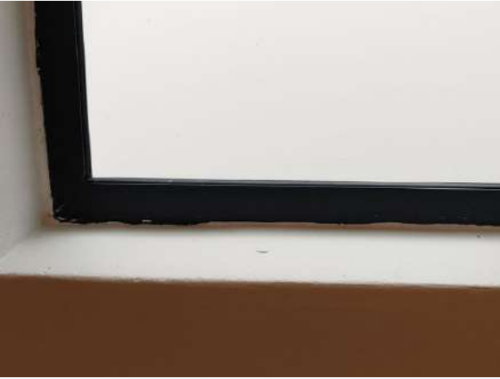
Ref # 21.2 - Untidy painting and finishing
