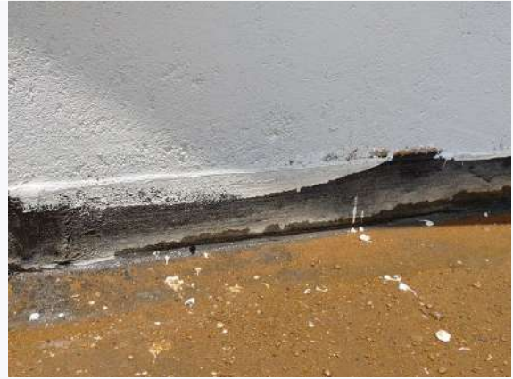
Ref # 4.2 - No cover flashing observed
