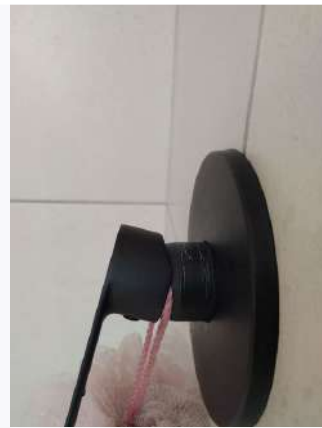
Ref # 18.6 - Mixer has scuff marks
