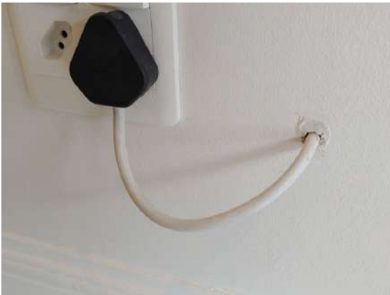
Ref # 15.1 - Hole drilled through wall for electrical flex cable
