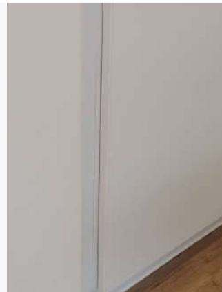
Ref # 11.4 - Cupboard doors and hinges require alignment and/or adjustment
