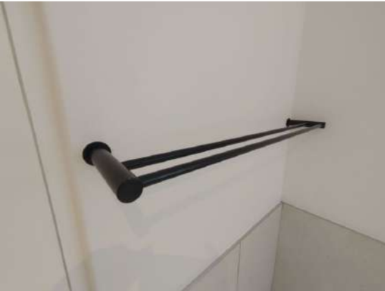
Ref # 20.1 - Towel rail is loose
