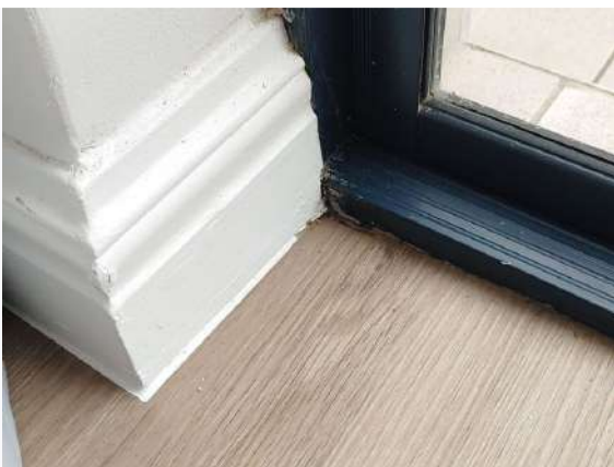
Ref # 10.1 - Untidy finish and no laminated cover strip
