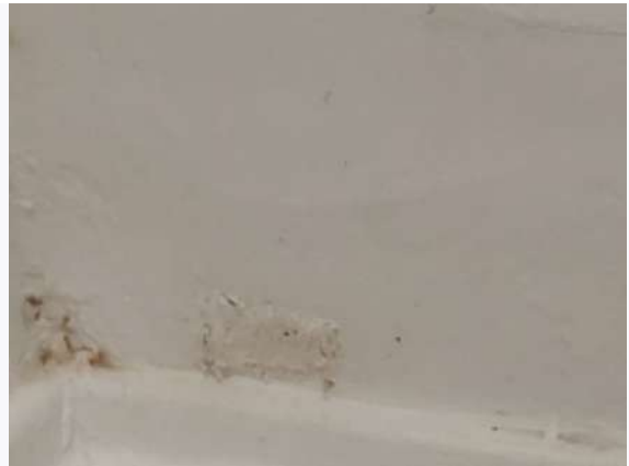
Ref # 21.1 - Wall with efflorescence
