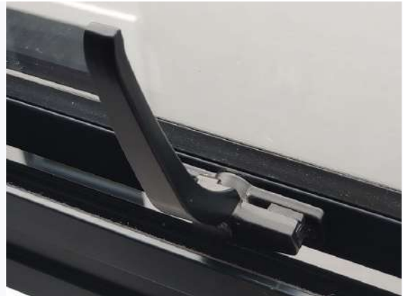
Ref # 11.2 - Window opener loose and requires adjustment
