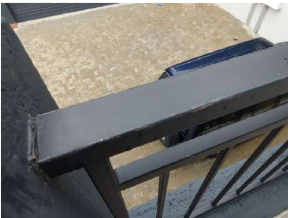
Ref # 12.1 - Rust observed on balustrade
