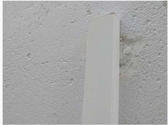
Ref # 2.1 - Untidy finishing
