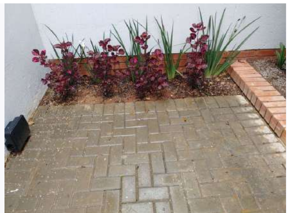
Ref # 23.3 - Weep holes for water run-off drainage is blocked and / or inadequate
