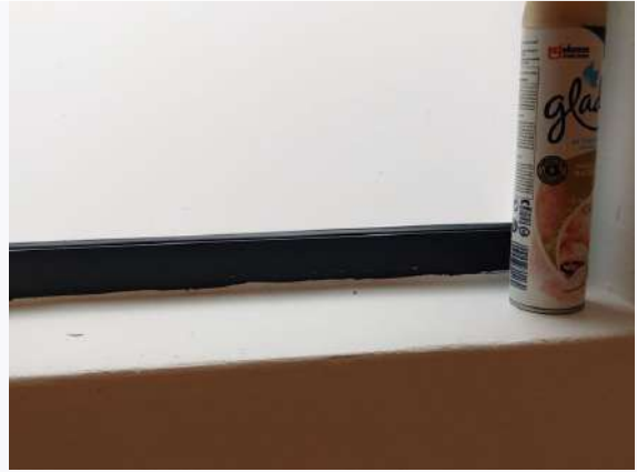
Ref # 21.2 - Untidy painting and finishing
