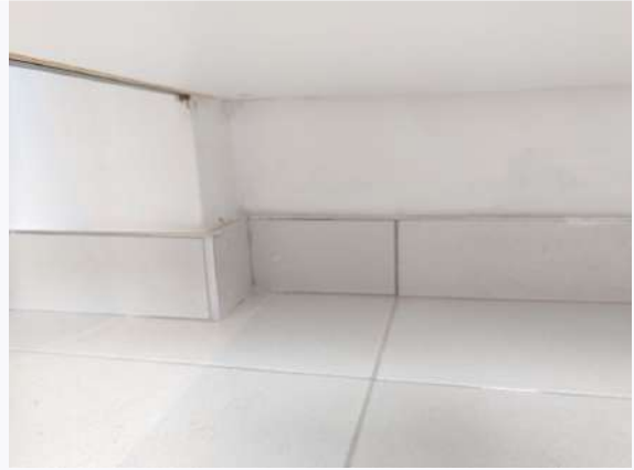
Ref # 18.1 - Untidy finishing
