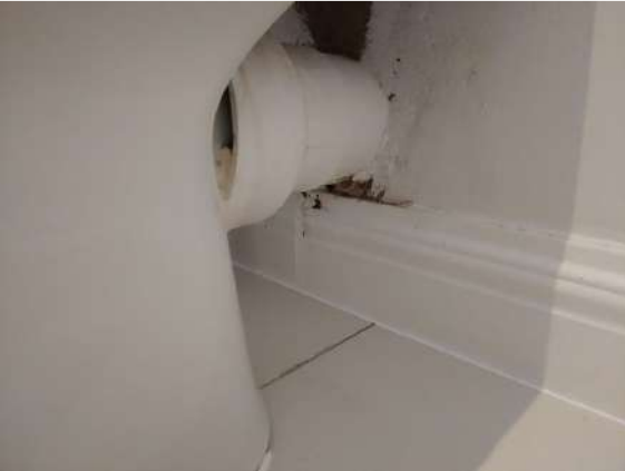
Ref # 21.5 - Untidy finishing behind the toilet and outlet pipe
