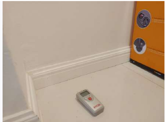
Ref # 15.1 - Active rising / lateral damp measured
