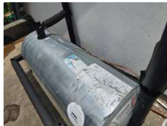
Ref #6 - Electric Geyser with Tank
