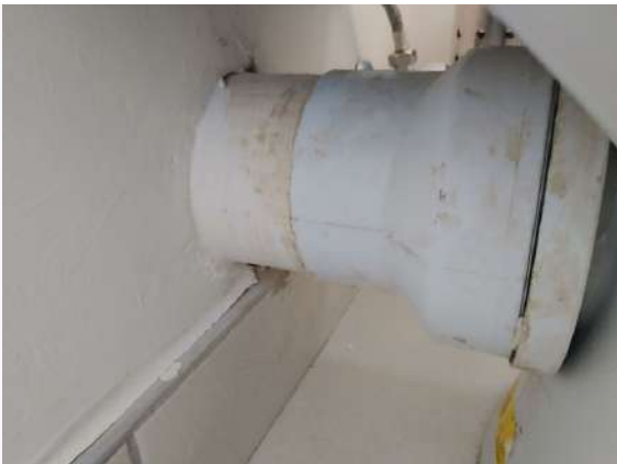
Ref # 19.3 - Untidy finishing behind the toilet and outlet pipe
