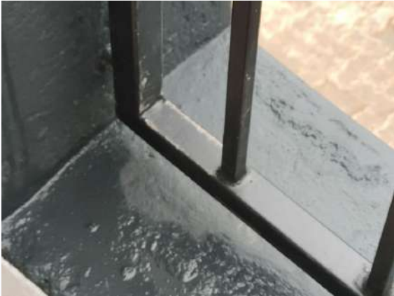
Ref # 12.1 - Rust observed on balustrade
