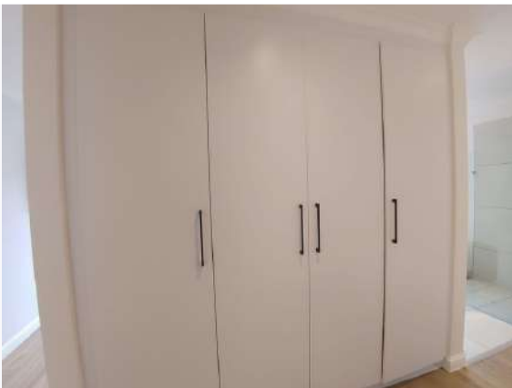
Ref # 10.4 - Cupboard doors and hinges require alignment and/or adjustment
