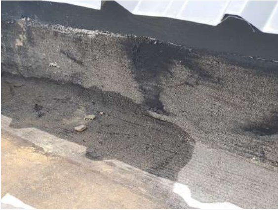
Ref # 4.2 - No cover flashing observed
