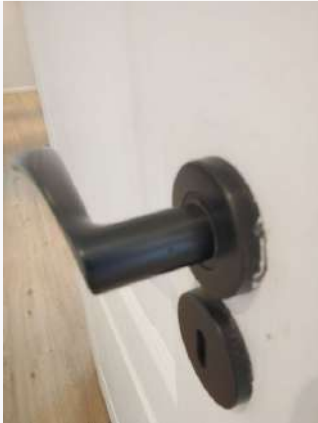
Ref # 10.3 - Paint splatter and scuff marks on the door lock sets
